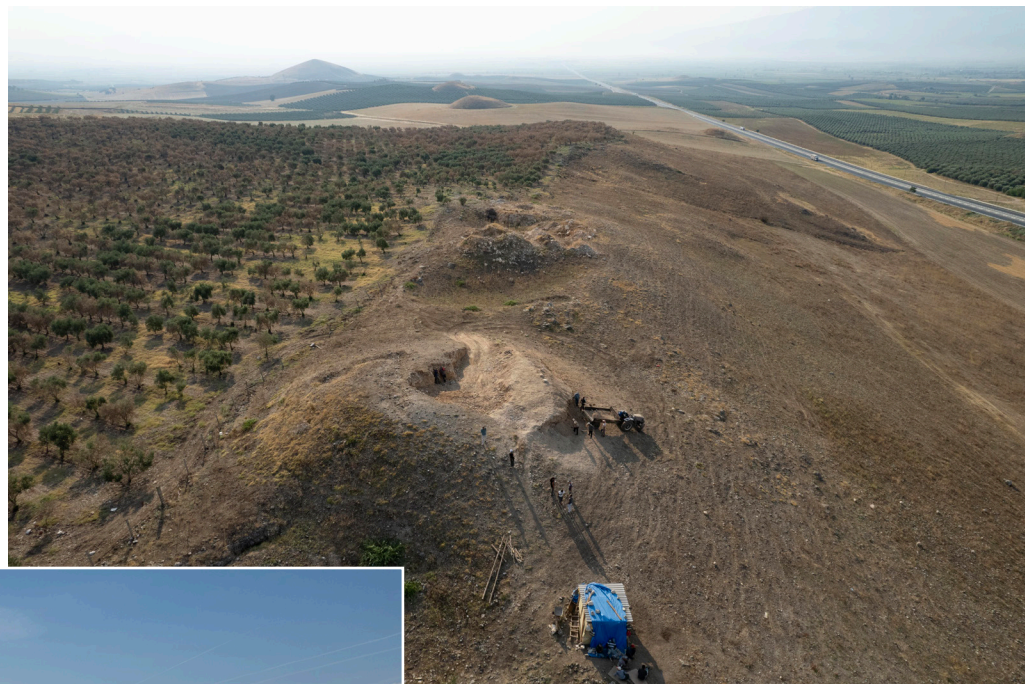
Fig. 1. Bin Tepe: View of progress of restoration of Tumulus BT05.026 in foreground with Tumulus of Alyattes on horizon in background.
