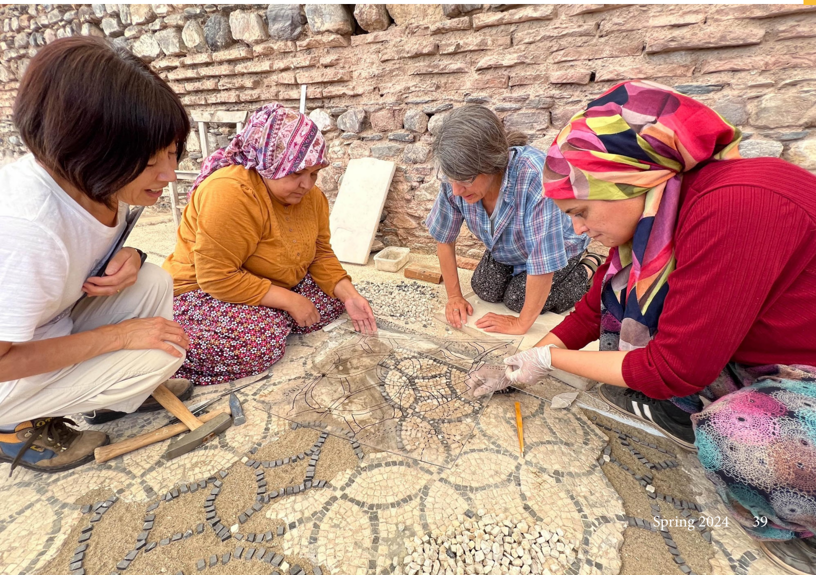
Fig. 4 Left to right: Hiroko Kariya (conservator), Emine Altan (local site preservation team), Catherine Alexander (illustrator), and Sevinç Akça (local site preservation team), restoring mosaics of the main hall of the ancient Synagogue at Sardis.
